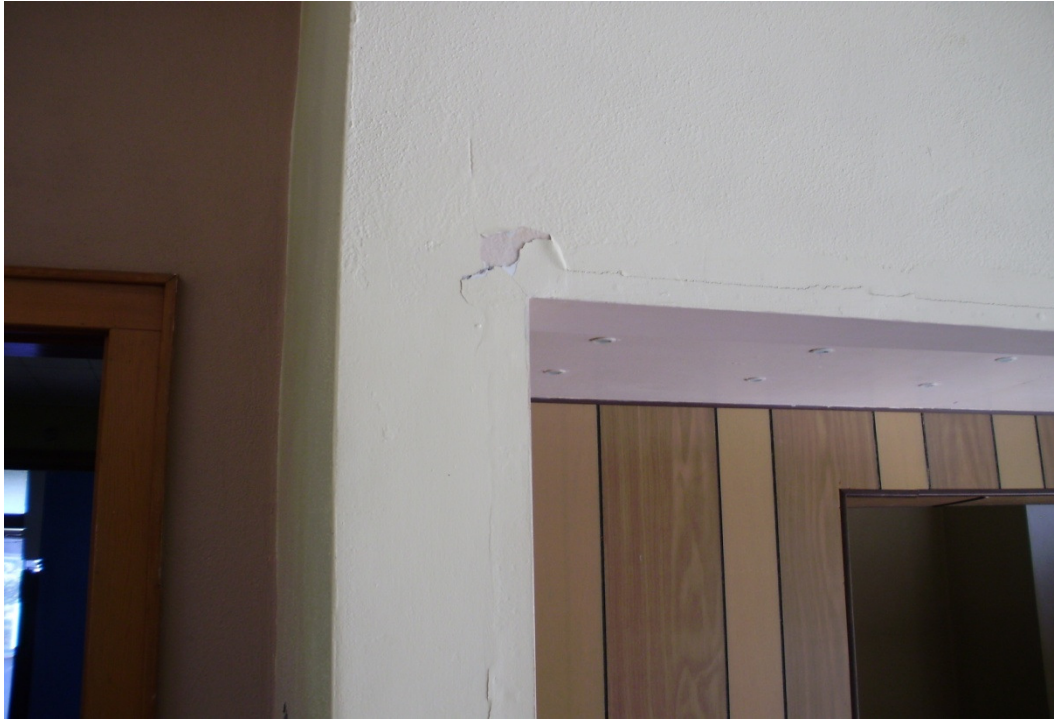
Photo 5: Room No. 9, AC mud joint compound (MJC) in the original building. Deem all MJC in this portion of the building to contain asbestos.
