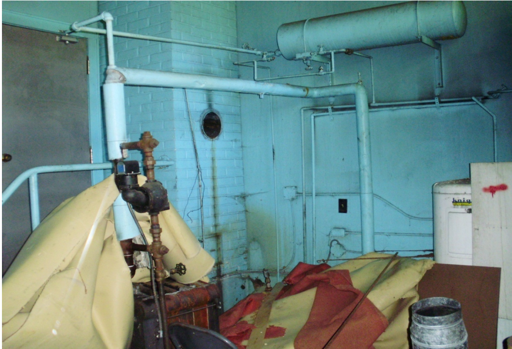
Photo 3: Room No. 18, AC air cell pipe insulation. Approximately 20 linear meters and 2 elbows. Unknown if it continues under building.
