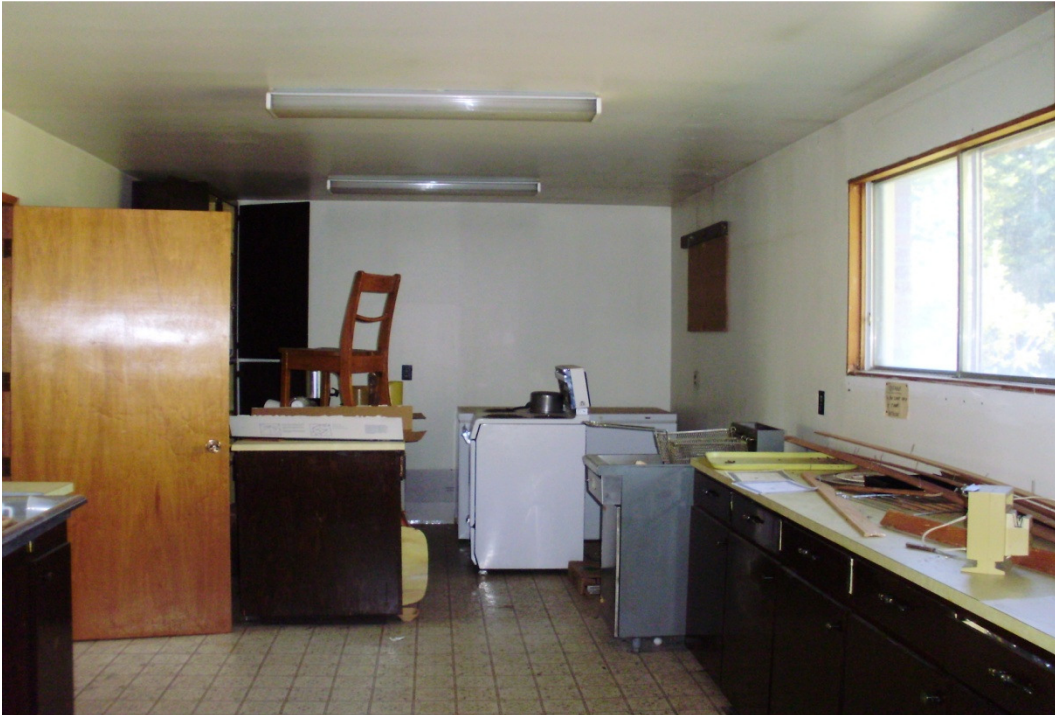
Photo 2: Room No.8, AC floor tile and possible freon containing freezer.
