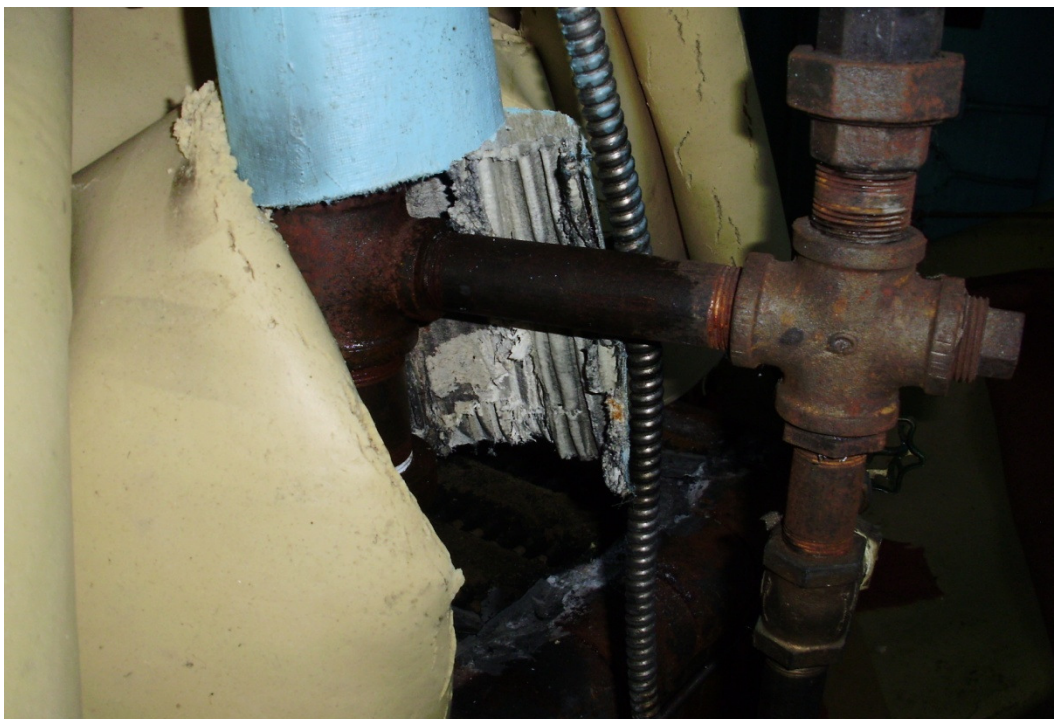
Photo 4: Room No. 18, AC air cell pipe insulation referenced in in the previous photo.
