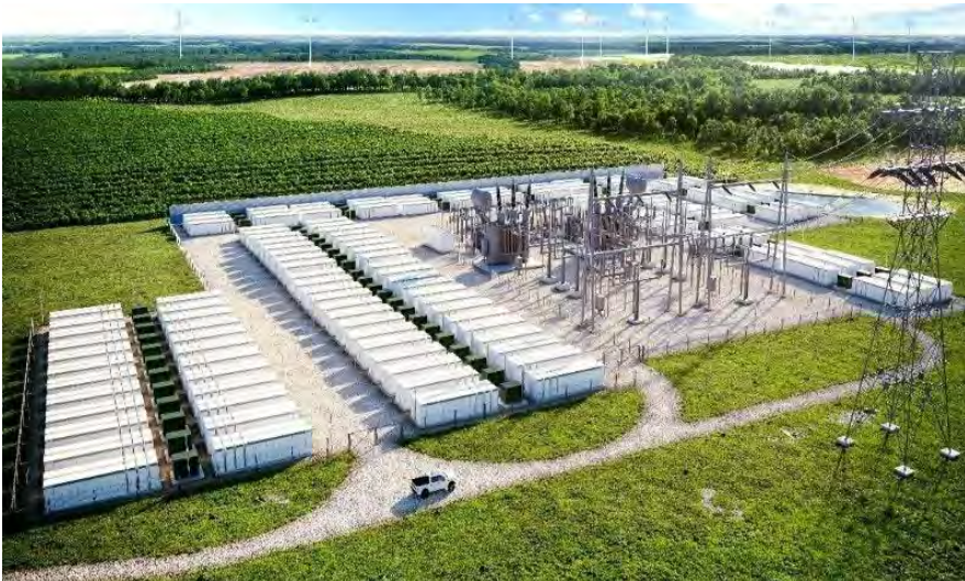
Example BESS site
